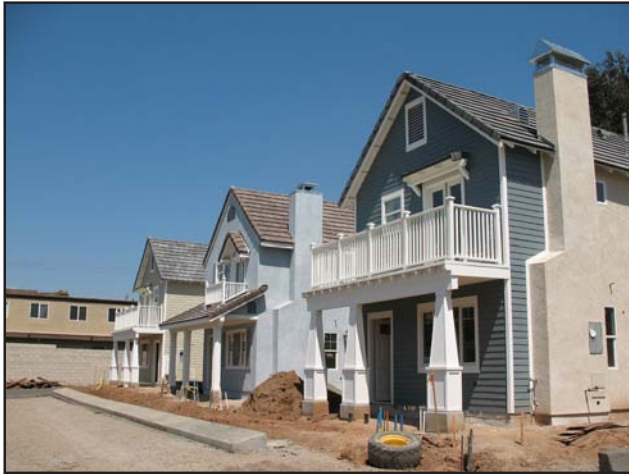
The exterior of the units at Wisconsin Cottages is now complete and landscaping is underway.
